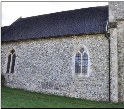
There are just two C14 Gothic Decorated style windows in the north wall of the nave. The western one is original whereas the eastern one is an 1863 restoration.
